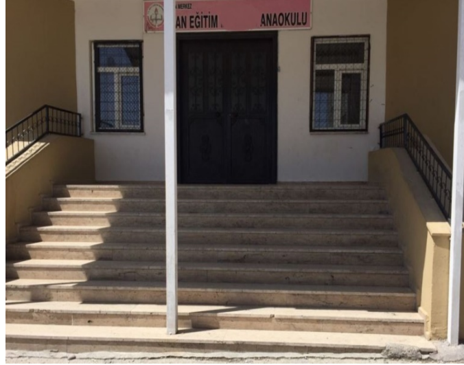
Figure 2. Star building school entrance without disabled stairs
